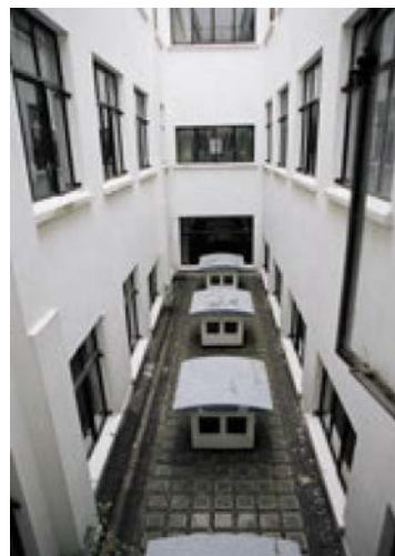
Figure 82 Exhaust fan units in 2005.
