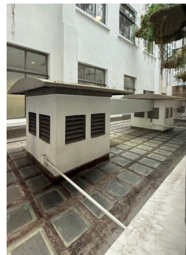
Figure 83 Exhaust fan units in 2025.
